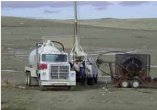
Production well service at in-situ leaching facility.
